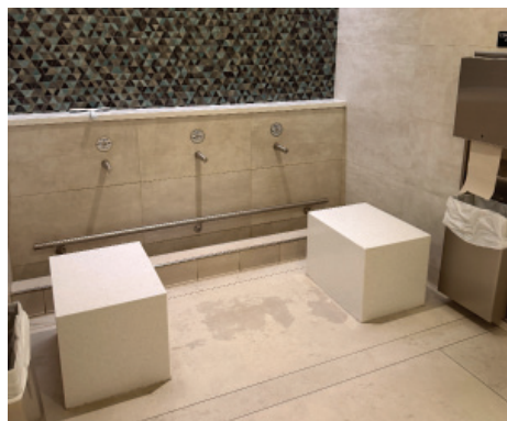
A washing station at George Bush Intercontinental Airport in Houston.
